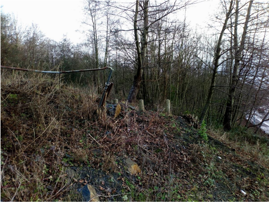
Obstruction and concrete bollards near Cwm Level Road between points A and B
